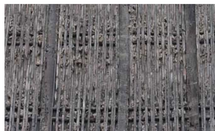
Figure 10. Examples of quincha dividing wall, Lima city centre. (Authors: Cristini & Ruiz Checa).
