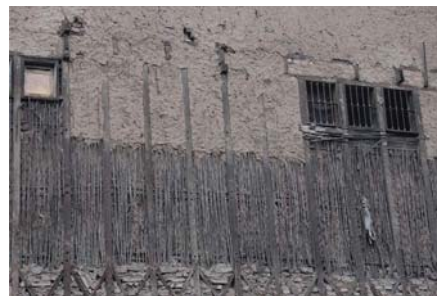
Figure 11. Details of the wicker screens, filled with earth, in a quincha wall, Lima (Authors: Cristini & Ruiz Checa).
