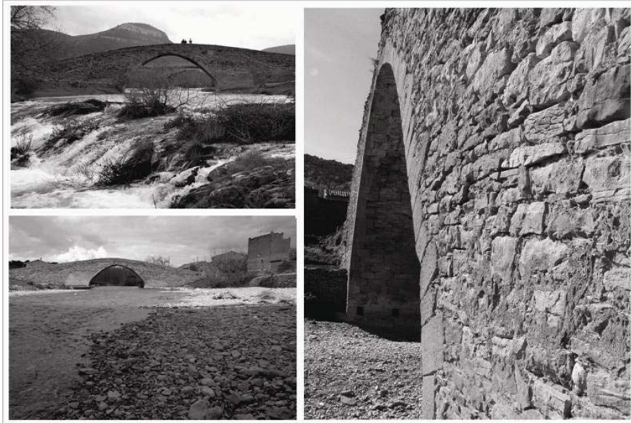
Figure 6: Images of the Pobleta de San Miguel Bridge, built with ashlar's masonry and dry stone
