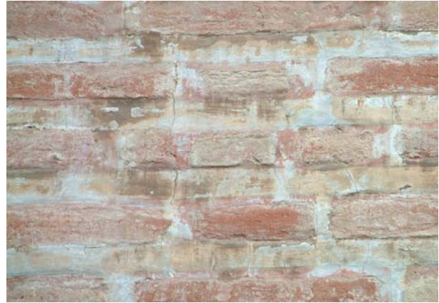
Figure 9. Detail of the fake brick wash treatment on the palace rear facade
