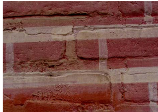
Figure 3. Aduana Palace- 1758-70. Detail of the original fake brick wash and the recent restoration (1996-1997)
