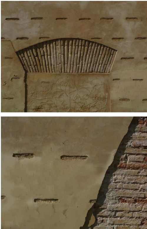
Figure 7. A surface detail, simulating header bricks. Palacio del Gremio de Carpinteros (Ancient Carpenters' Trade Centre) (Authors: Cristini & Ruiz Checa).
