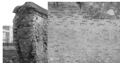
Figure 6. Details of Type 2-wall. Section of the fencing of San Miguel de los Reyes; Elevation Mascarell city-wall, Valencia (authors).
