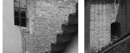
Figure 8. Details of Type IV-wall. Elevation of the Farmhouse of Falco, Godella; Elevation of Saint Ursula Church, Valencia (authors).
