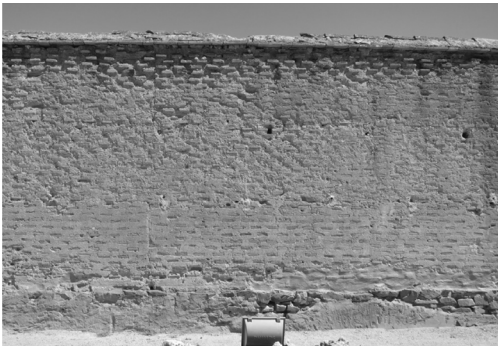
Figure 1. Brick-reinforced rammed earth wall; fencing wall of la Cartuja del Puig, Valencia (authors).
