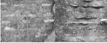
Figure 7. Details of Type III-wall. Detail of the elevation of Convent of San Diego, Alfara Patriarca, Valencia; detail of the elevation of the fencing, Carabona Tower, Burriana (authors).
