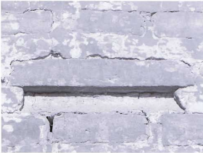
Figure 3. San Andrés church. Detail of the double joints in the masonry of the front of Calle Procida. First part of 17th century
