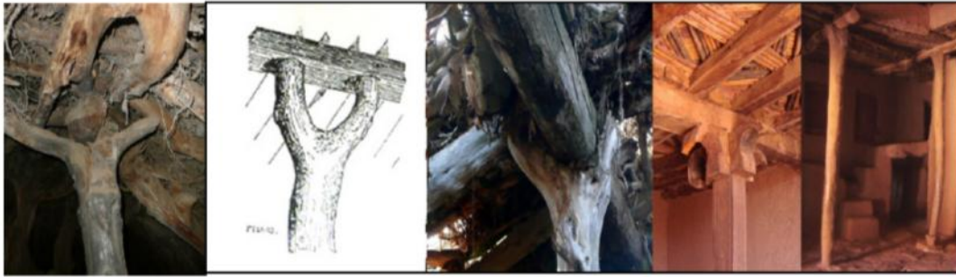
Fig. 4. Different types of “pitchfork” structures, from the left: Viollet le Duc drawing, chozones supports, some examples of vernacular architecture in Morocco. (Ruiz – Cristini).
