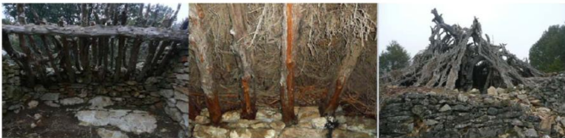
Fig. 6. Different stages of the thatching of the roof by juniperus thurifera branches in shepherds shelters (Ruiz – Cristini).
